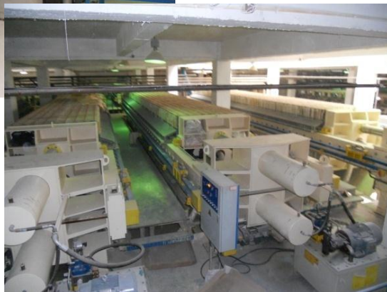
New filtration system
